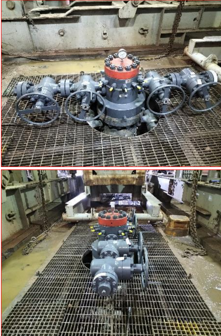
Figure 7. Maverick T463 A1-1 installed wellhead equipment photo.
