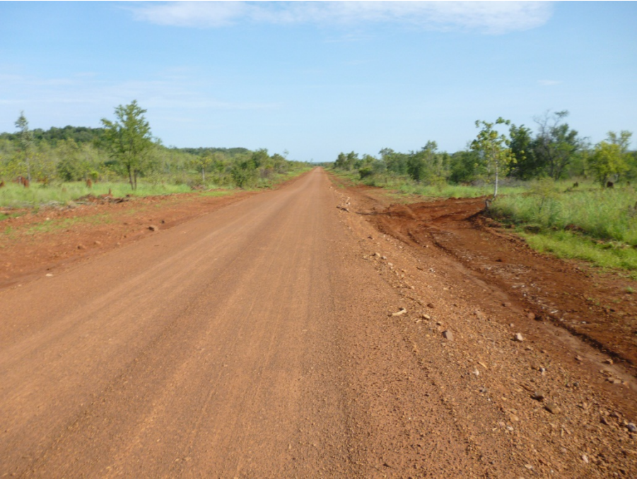
Section of the 10km x 6metre wide access road from the Roper Highway
