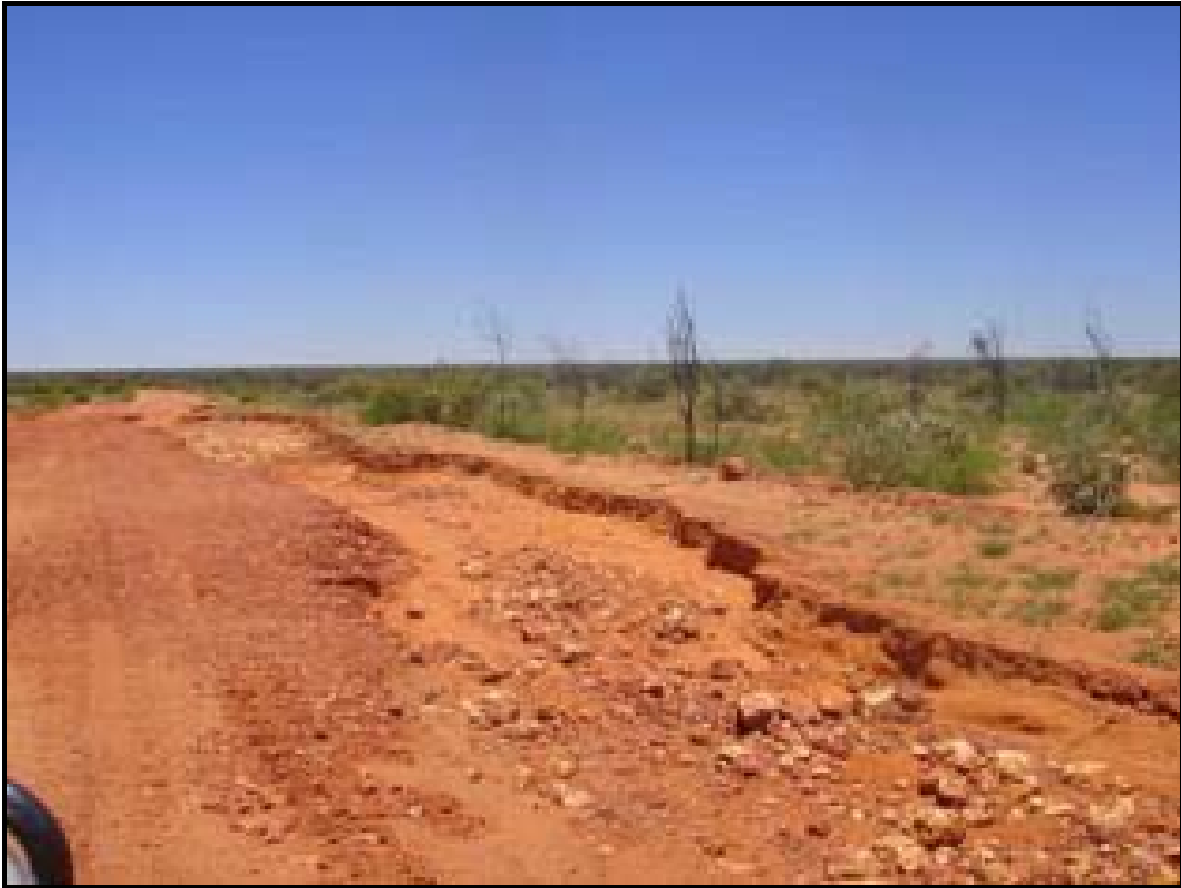
Photograph 1 – Typical area of previously formed road requiring repairs.
