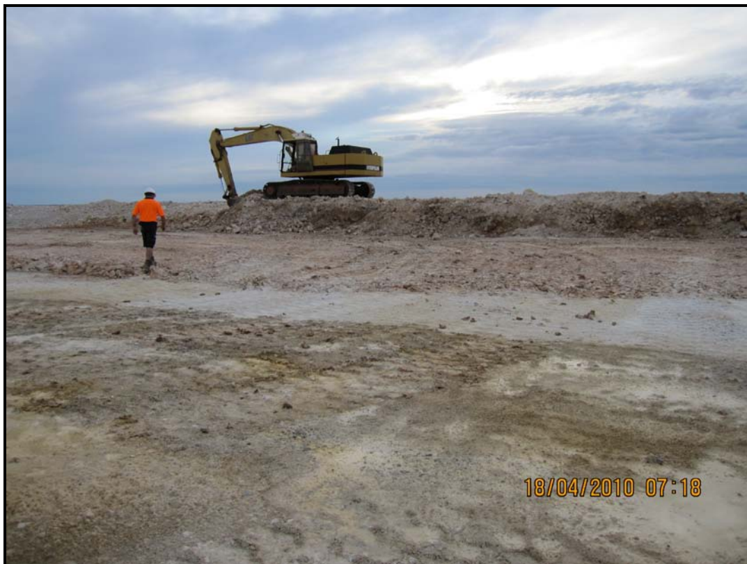
Photograph 6 - 200mm of BPH remaining on Waste Dump Floor.
