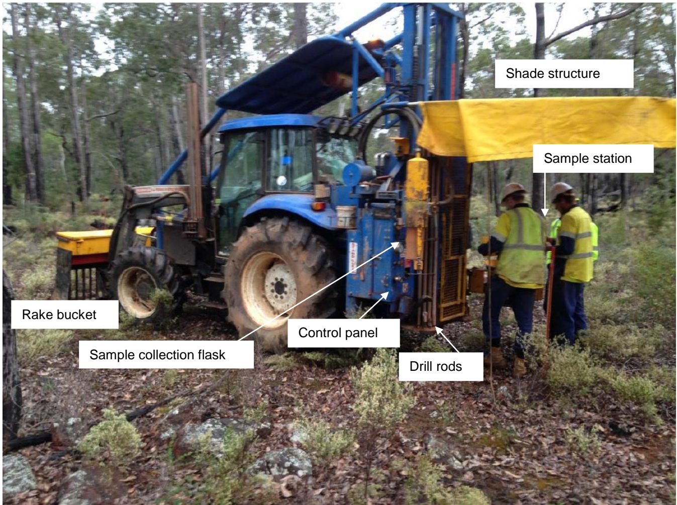
Figure 2. A tractor mounted vacuum drilling rig, of the type used, in uncleared forest
