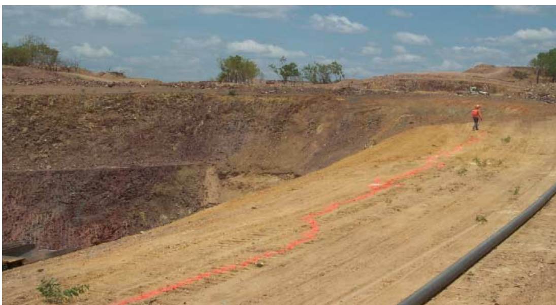
Figure 3.6.1. Cracks painted along the eastern wall of Millars.
