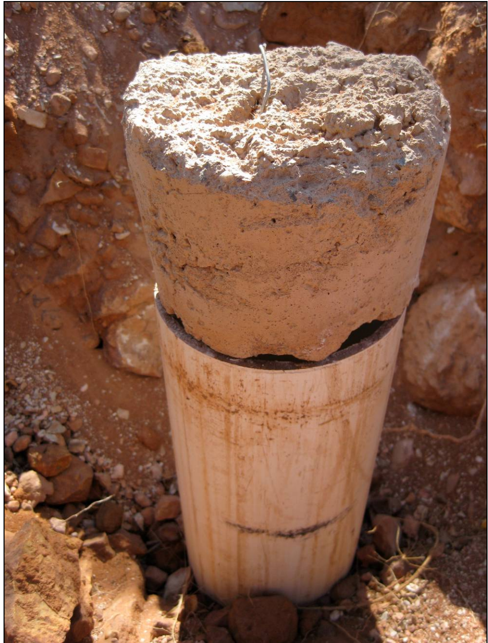
Plate 4.10 Inappropriate cap on drill hole.
