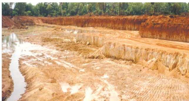
Figure 40.13. One of the open pits at AN47 quarry. Excavation is down to water table (photograph from Doyle 2001).
