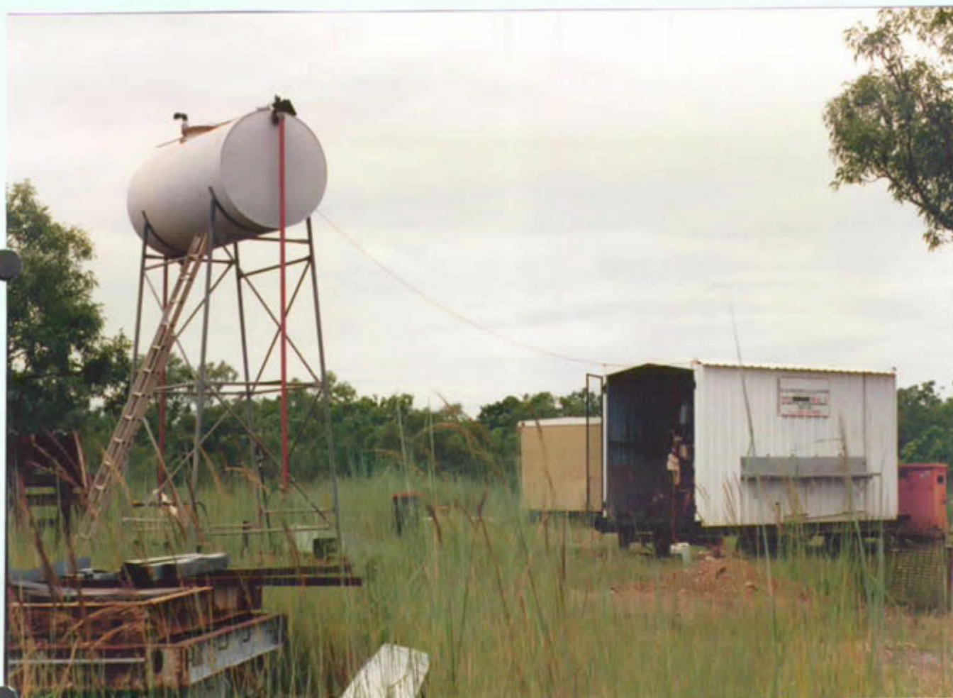
FUEL TANK AND POWER GENERATOR ON MCN-4187.
