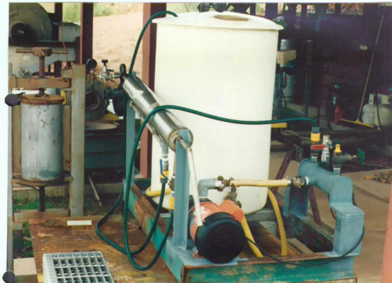
MERCURY RETORT AND PRESSURE FILTER IN POSITION.
