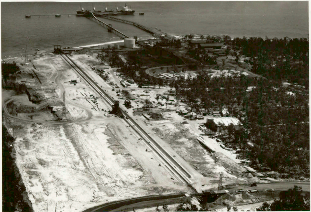
View of new stockpile area taken in August 1971. Erection of stacker and reclaimer taking place in centre. Dumping hopper in foreground.
